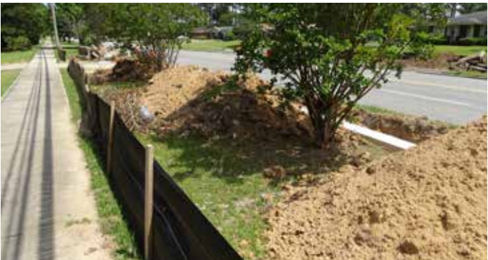
Trenching for utilities severs tree roots and destabilizes trees. The city could require boring or tunneling for utility installation instead.
